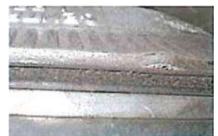
Signs of overheating
